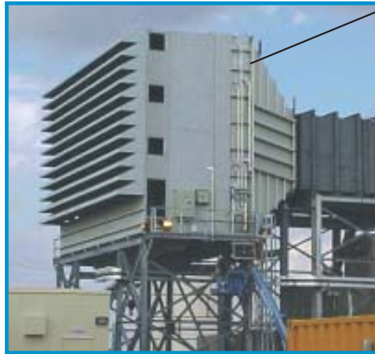
Evaporative cooler section is typically located behind filter section
