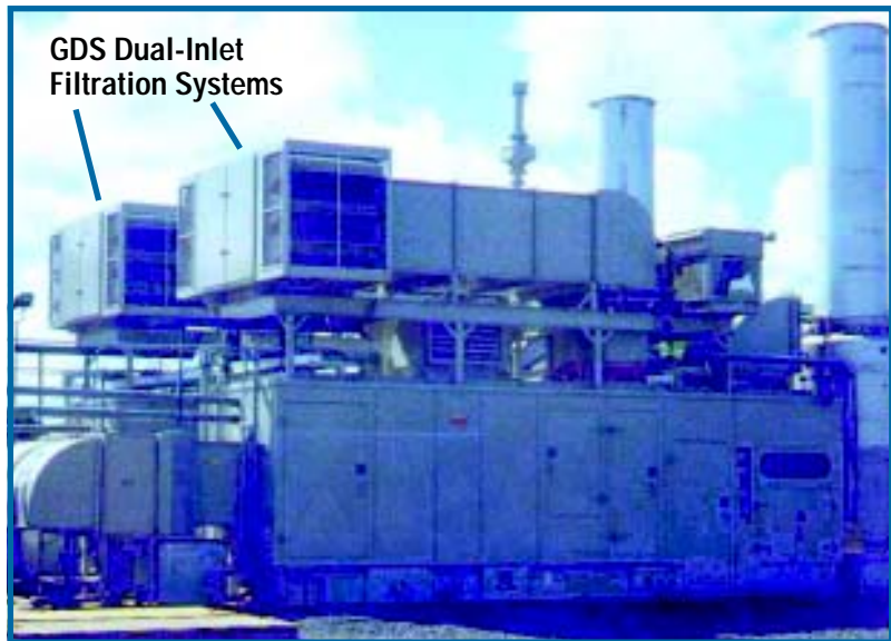
These Donaldson Dual-Inlet GDS Filter Systems protect turbines from the ravages of sand and dust near Tucson, Arizona USA. Note the insect screens over the inlet hoods. Donaldson GDS systems keep combustion air clean for hundreds of turbines all over the world.
