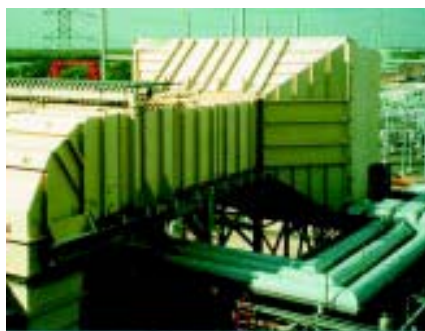
Donaldson often provides the ducting to the turbine along with the filter, as shown in this photo of the GDX at San Antonio, Texas USA
