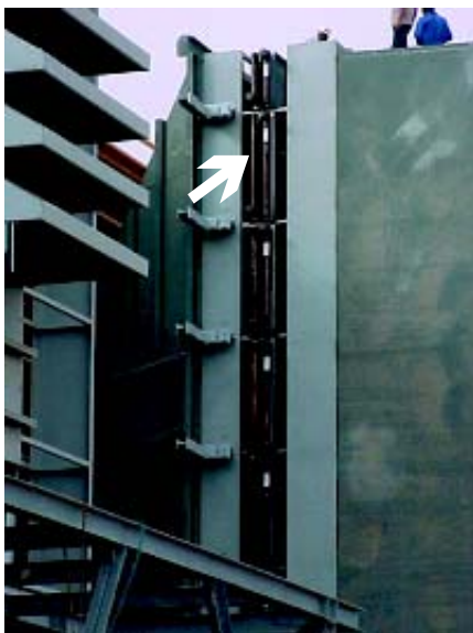
The Donaldson Chiller Coil System typically occupies the space between the filter house and the transition.
