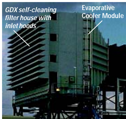
This Donaldson Evaporative Cooler enables this GE Frame 7FA Gas Turbine near Lubbock, Texas, USA, to yield maximum output even during the hot dry summer months.
